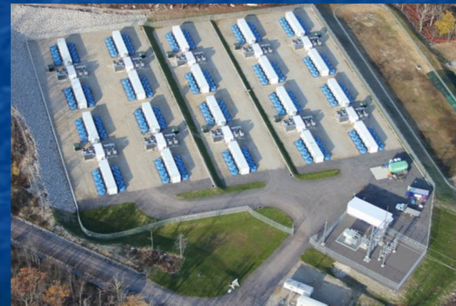
The flywheels are buried in the ground to reduce visual impact and run silently
